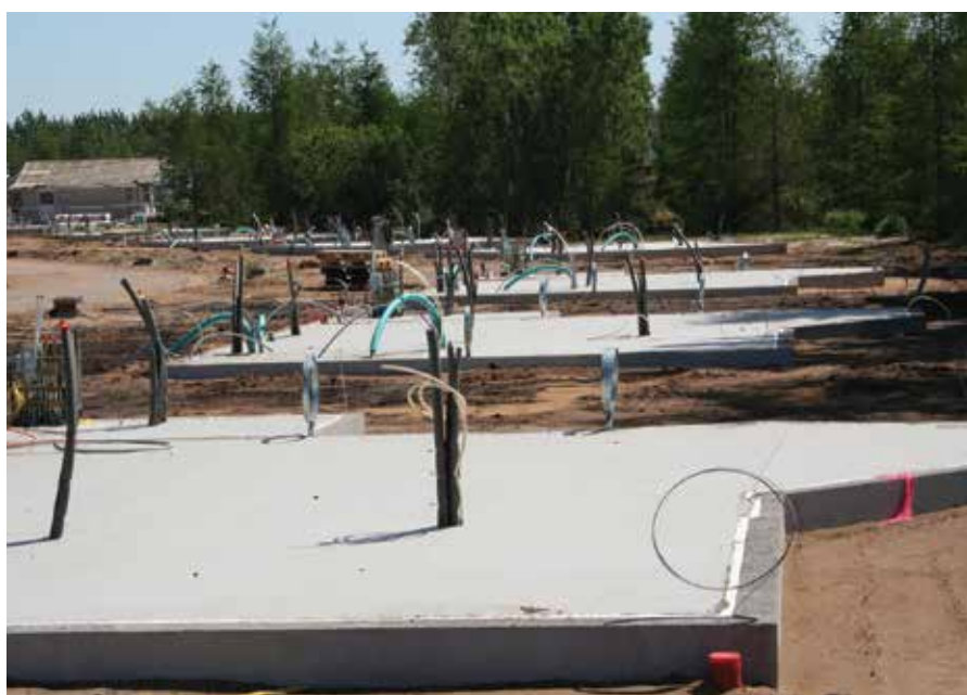
Termix distribution units for floor heating are installed in each holiday house.
