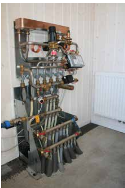
The Termix VMTD "Lalandia" substation is a complete unit for controlling the district heating installation in a house.
